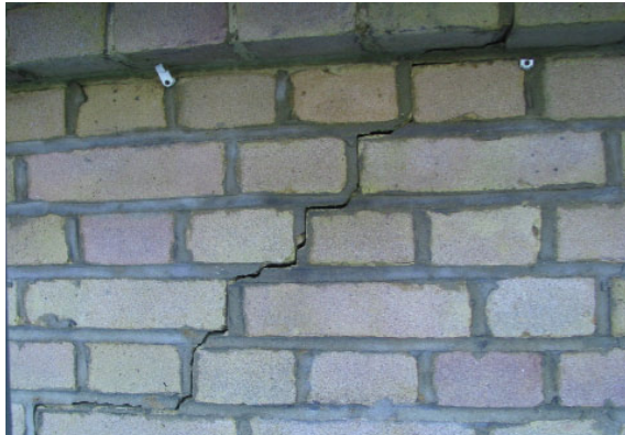
Existing cracks visible after cleaning (north elev)
